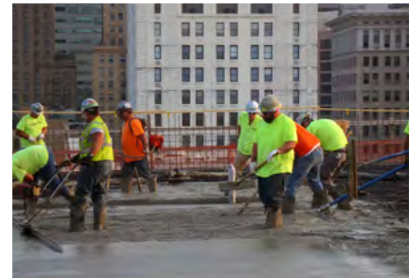
Crews work on final concrete pour for GE Building which topped out in June.
