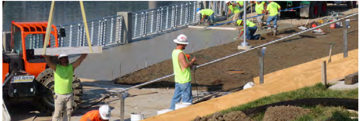
Crew installs granite steps and executes a concrete pour for the Ohio River Walk.
