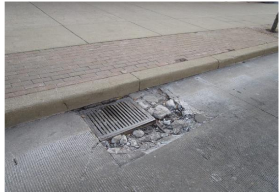
Figure 1. Cracked concrete around drainage
