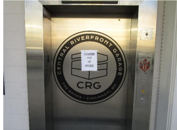
Figure 6. Elevator Out of Service
