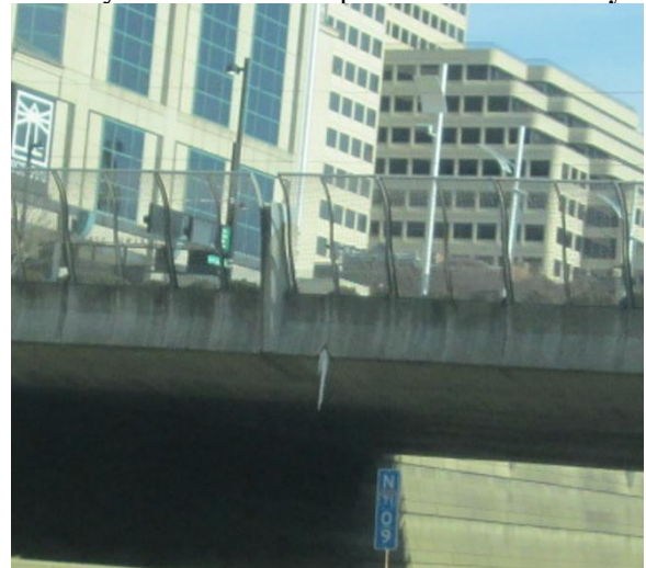
Figure 3. Icicle Formation on Bridge Fascias
