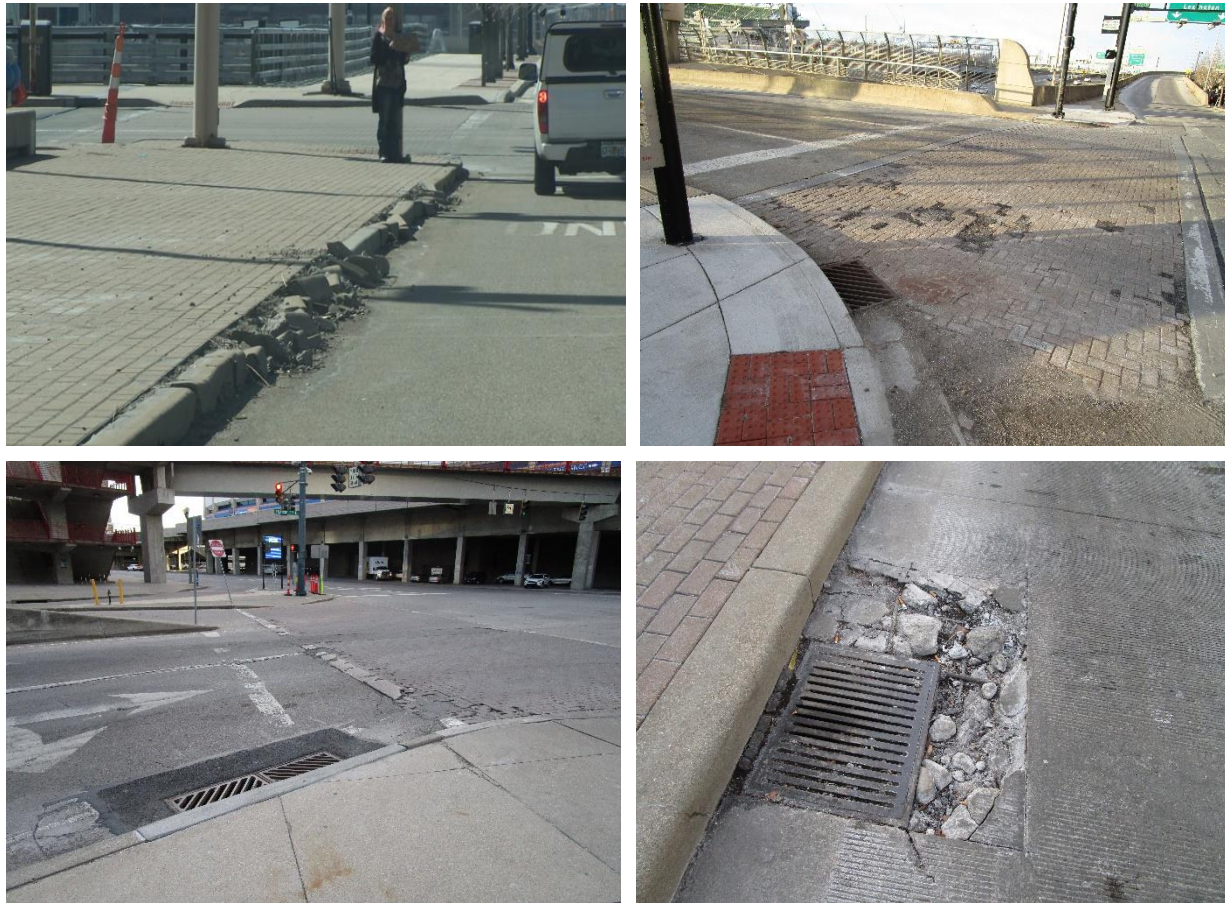
Figure 8. State of Repair Issues with FWW
