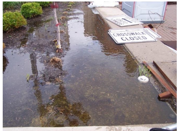
Figure 5. Project Site Flooding
