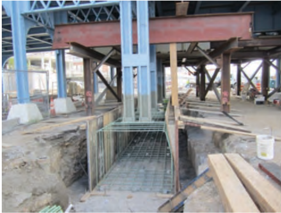
Photo #3 – Bid Package #9: Forming the last barrier wall under the Roebling Bridge approach.
