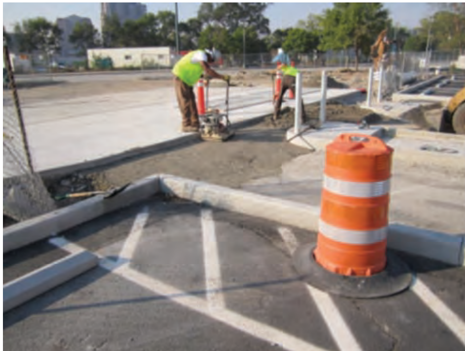
Photo #4 – Bid Package #9: Prep for pavement at the new Lot D entrance at Mehring Way.
