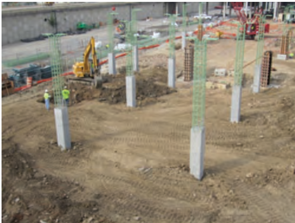
Photo #6 – Bid Package #11: The first columns on the south end of the Lot 2 Garage.
