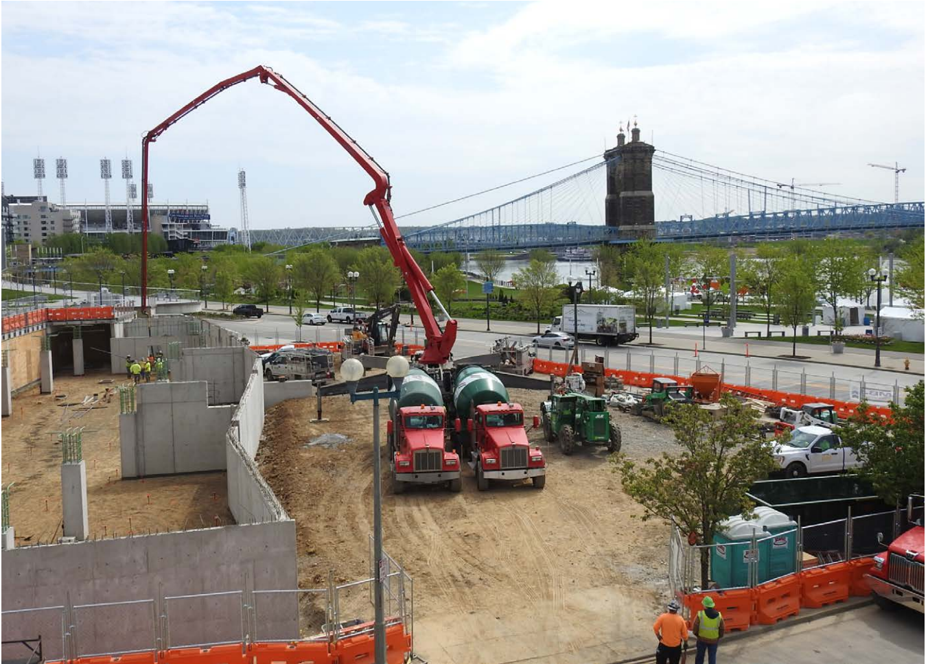
Workers orchestrate a slab-on-grade concrete pour at the future home of the Cincinnati Black Music Walk of Fame (Lot 28).
