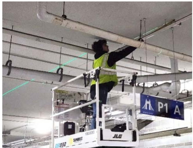
Parking guidance system installation gets underway in the Central Riverfront Garage (CRG). 🔗
