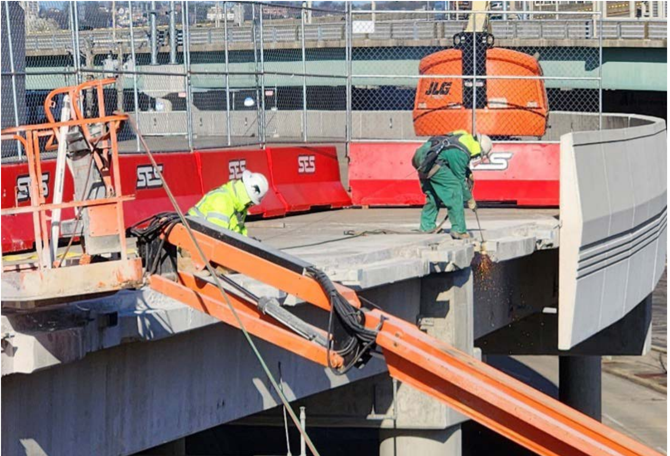
Paycor Stadium Plaza enters demolition phase prior to design improvements for greater access and smoother pedestrian traffic flow.
