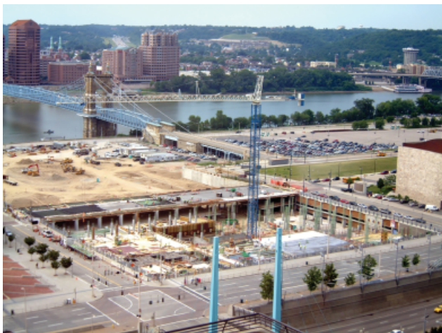
Figure 10. Parking structure and street grid under construction, demonstrating creation of the floodable parking structures supporting the raised street grid and podium, viewed from the northeast (July 2009)
